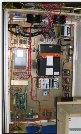
Before Power Supply/Drive Cabinet
