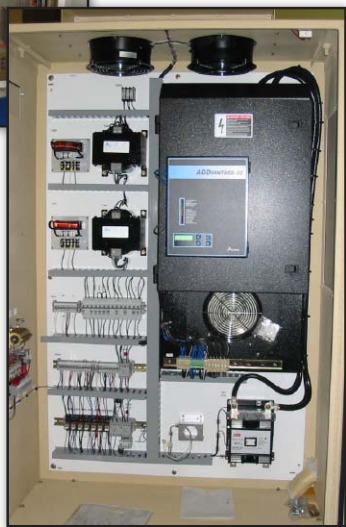
After Power Supply/Drive Cabinet
